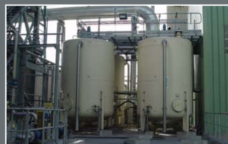
CTG La Réunion (Powerplant) Flue gas cleaning Zero Emission
